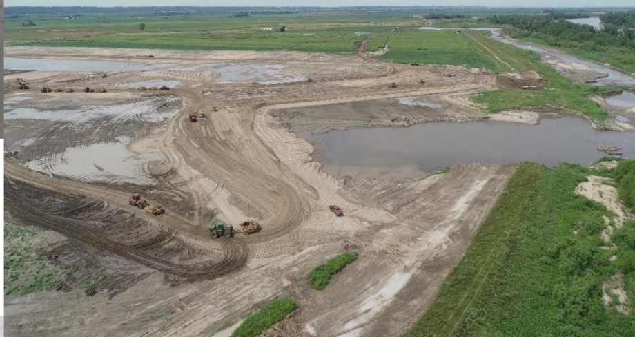
F Breach, July 2020 (with temp ring levee to prevent site from flooding)
